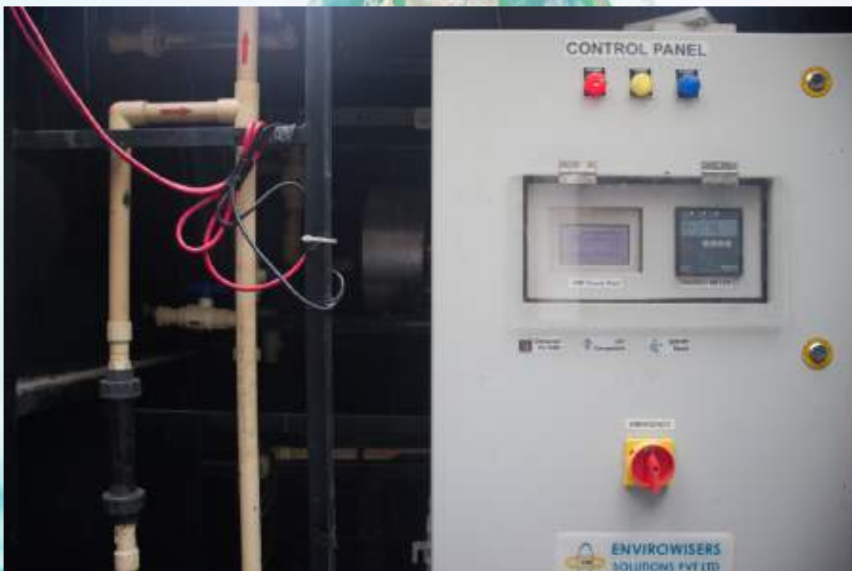
STP System at SSMRV
