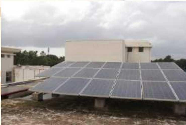
Solar pannels installed on rooftop
